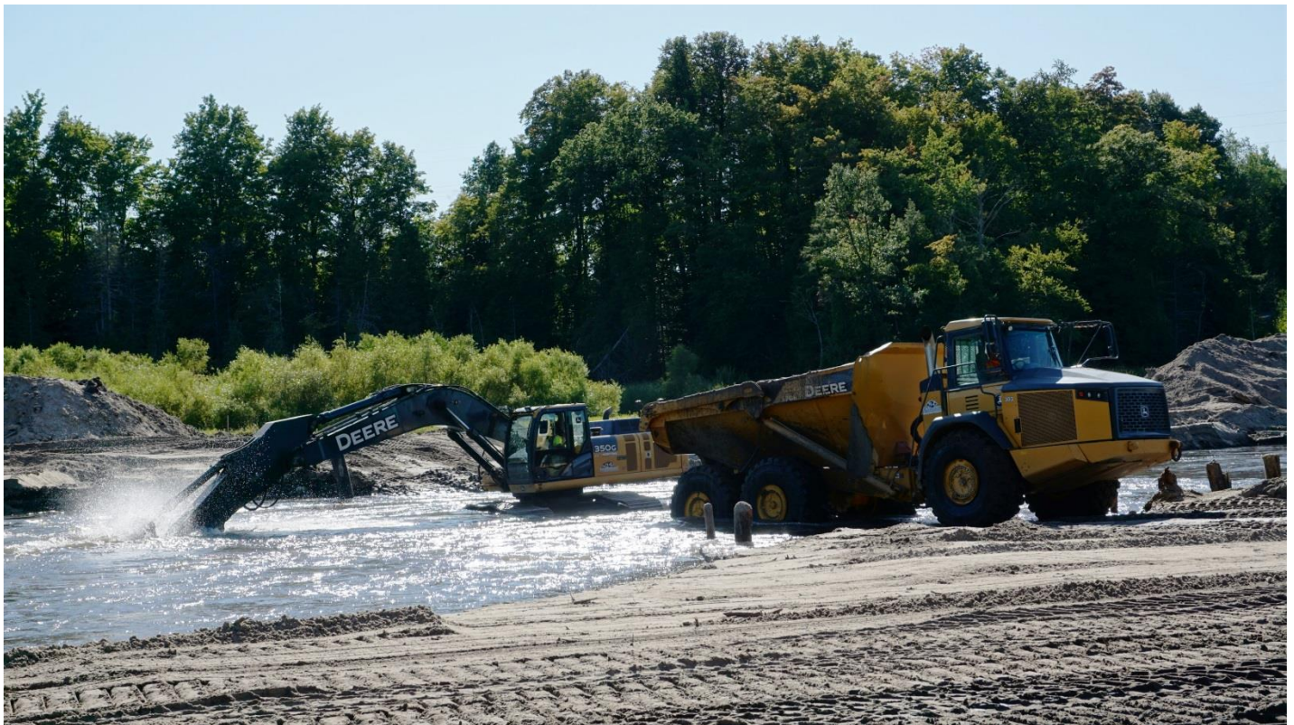
Off-road dump trucks with extra large tires back right into the water to collect sediment & haul it to a series of designated spoil areas that are outside of the reach of the future channel & floodplains.
