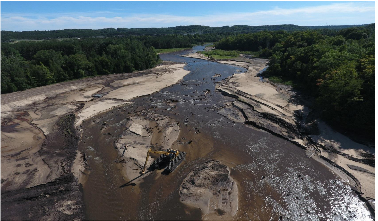
Aerial of channel excavation through exposed stump field, photo by GTB Natural Resources
