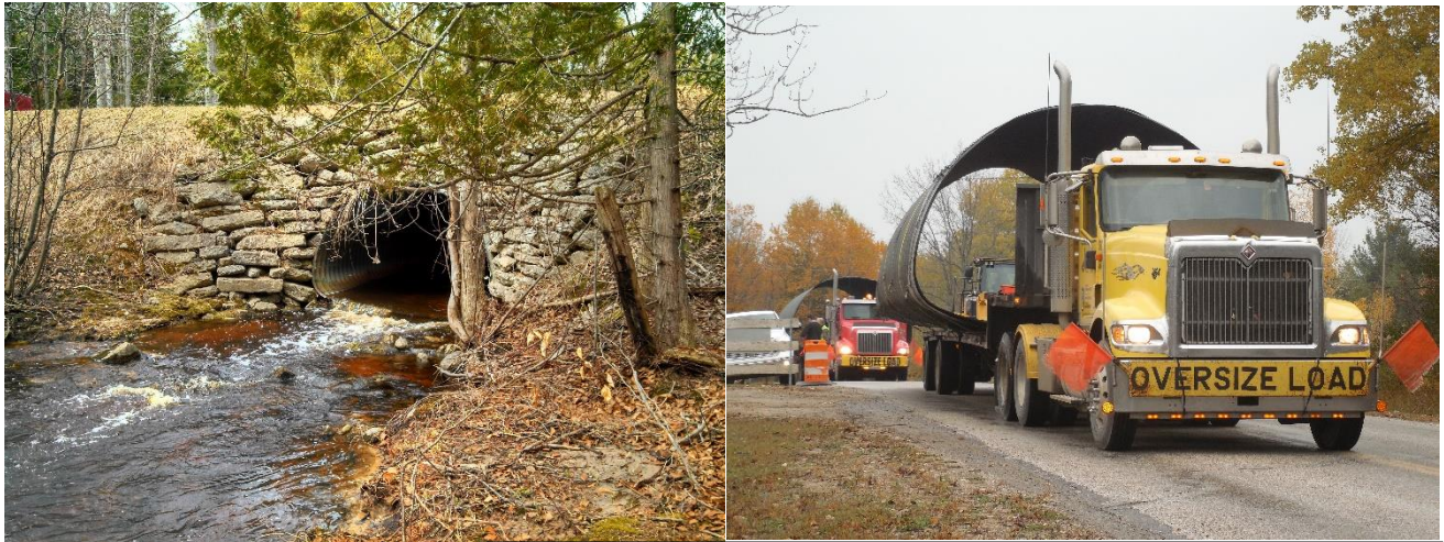
Left: Haynes Creek/Quick Road before replacement Right: Haynes Creek/Quick Road new culvert to be installed
