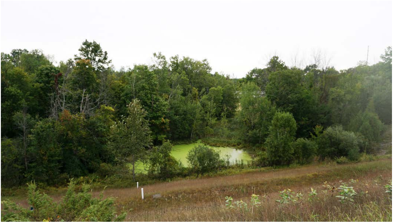
October 2016 – Standing on Boardman dam earthen embankment/concrete wall looking downstream to Cass Road Bridge, barely discernible behind trees. Standing water is evidence of seeps from original river channel.
