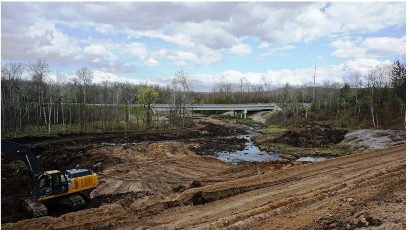
April 2017 – Getting ready to return the river to its original streambed; building the channel.
