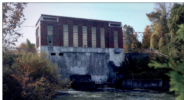
Record-Eagle file photo/Jan-Michael Stump The Sabin Dam was built in 1902 to provide hydropower to the region. It was decommissioned by Traverse City Light & Power in 2005 and now holds water in Sabin Pond in Garfield Township. It is scheduled to be removed after the Boardman Dam.
