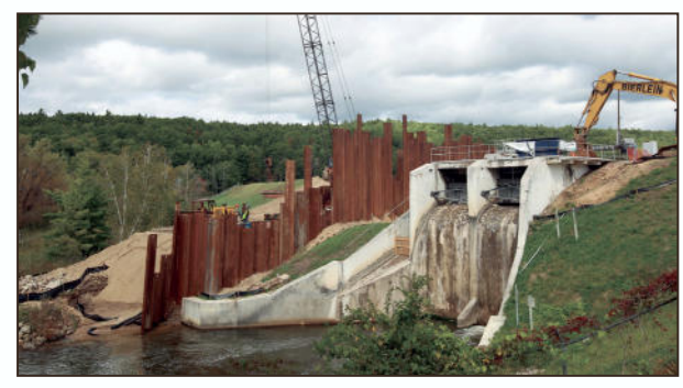
Record-Eagle file photo Brown Bridge Dam was built in 1921 to provide hydropower to the region. It was decommissioned by Traverse City Light & Power in 2005 and deconstructed in 2012, as shown above. Sandy soils underneath the dewatering structure gave out during dam removal, allowing water collected in a pond behind the dam to gush miles downstream, flooding many properties.
