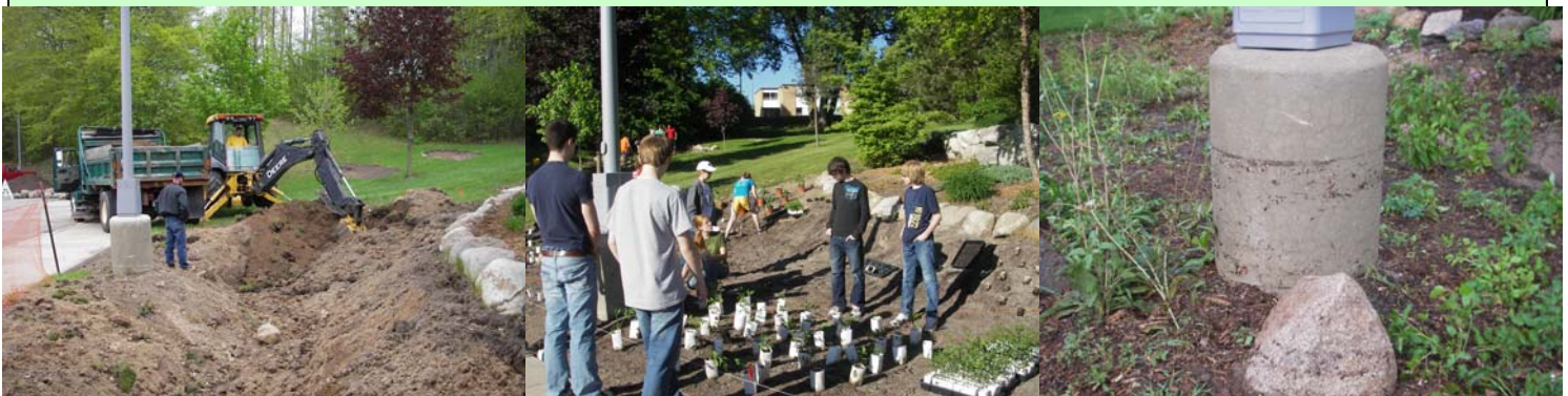
Pictured above: Construction of the rain garden, planting the rain garden, light pole showing the garden had been under 2 feet of water during the August 2 rain event (5—6 inches in an hour). The plants held firm.
