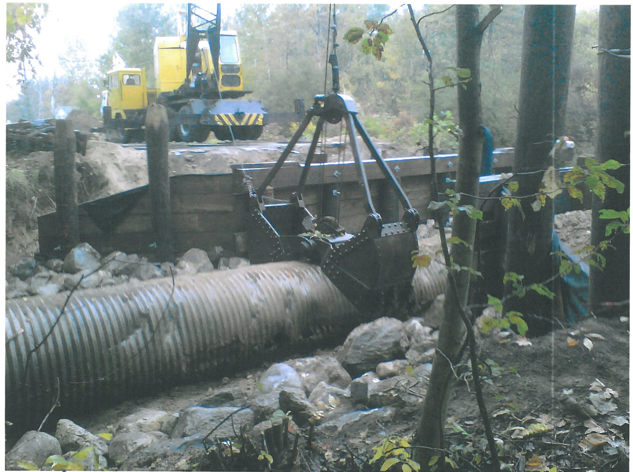
10.3.12 Carlton Creek - S. section of culvert in process of being lifted out of stream flow
