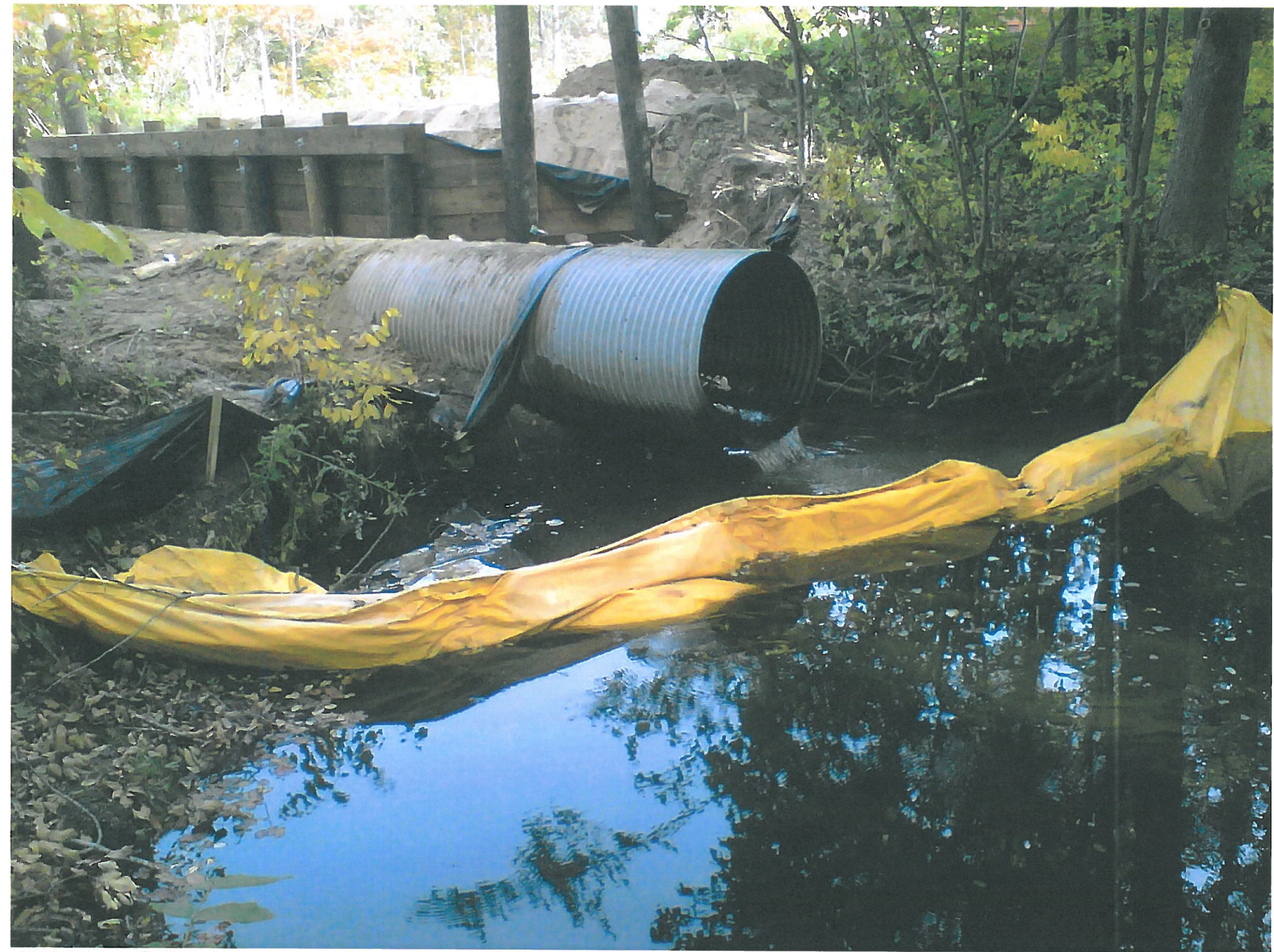
10.1.12 Culvert view from S.W. side of scour hole on Carlton Creek @ Arthur Road
