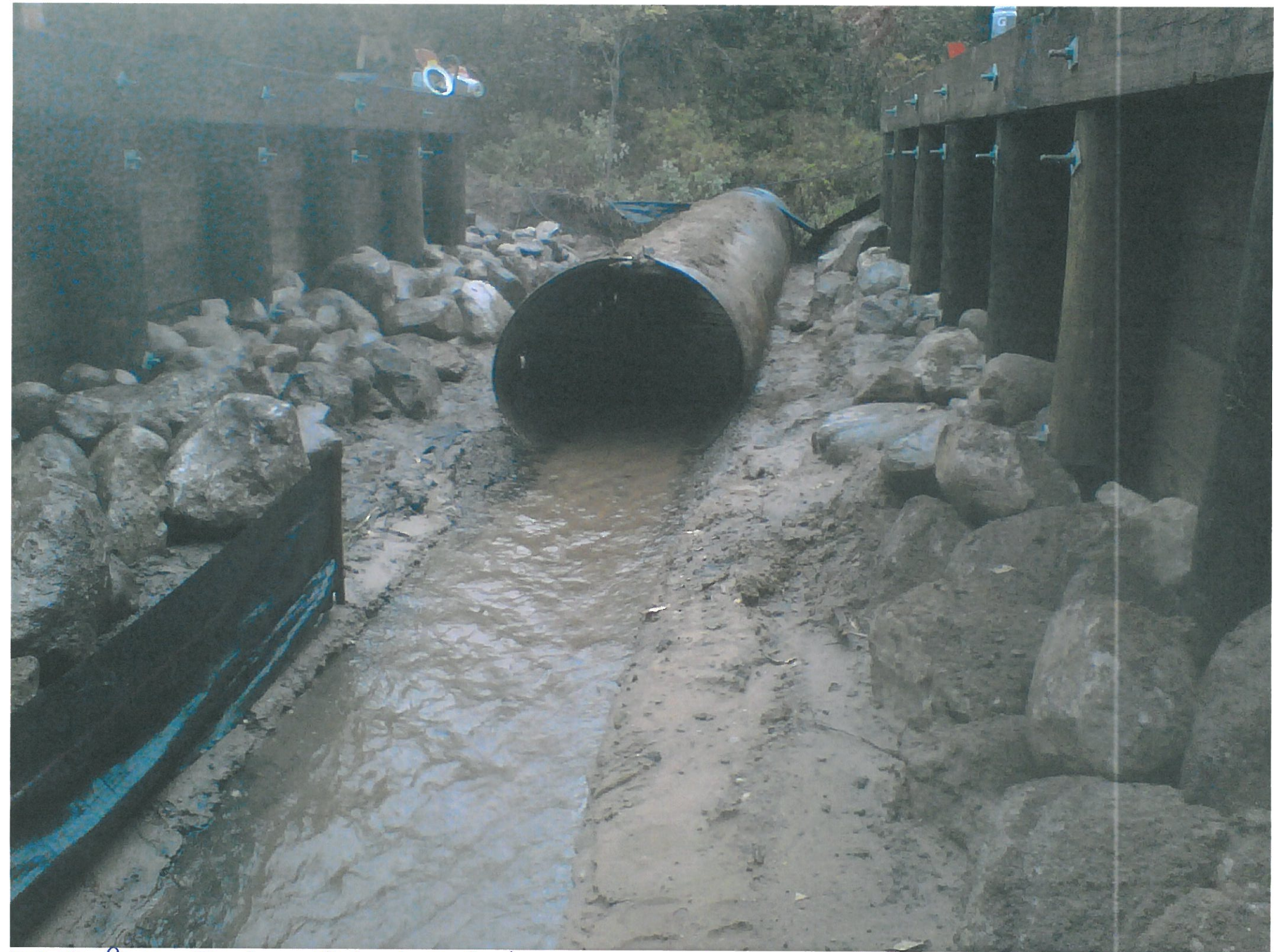
10-3-12 Carton Creek Culvert section to S. removed: n. section prior to removal
