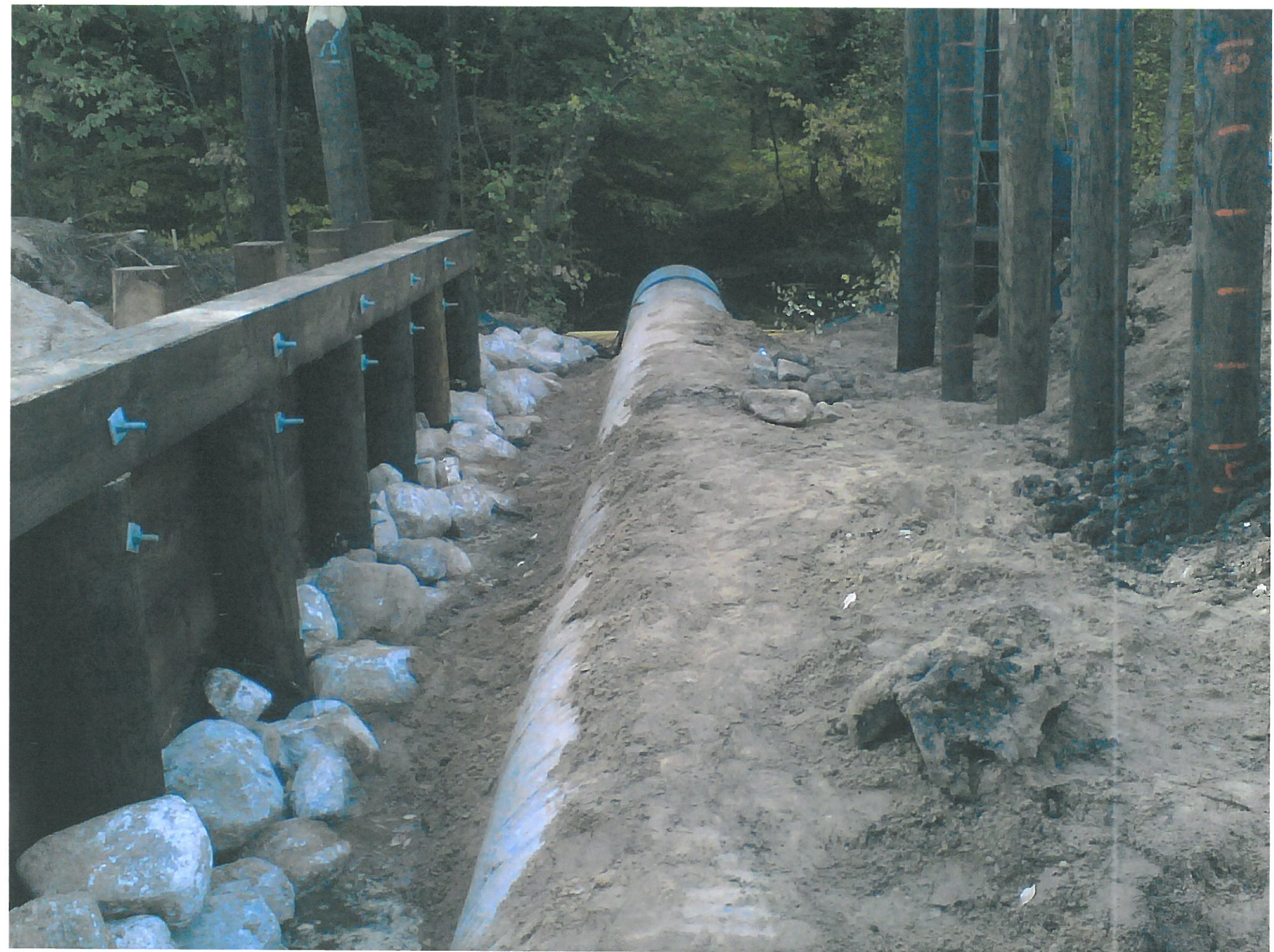
10.1.12 East Abutment and heavy rip-rap complete; piling to be driven today @ west (right)
