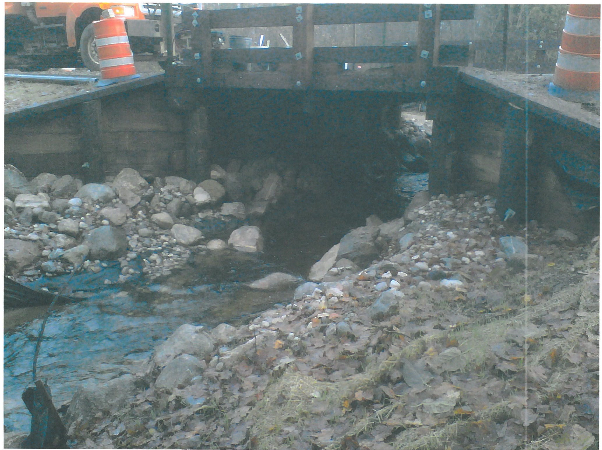
10.24.12 View of new timber structure from s.e. ; note grass has rooted nicely in straw mat
