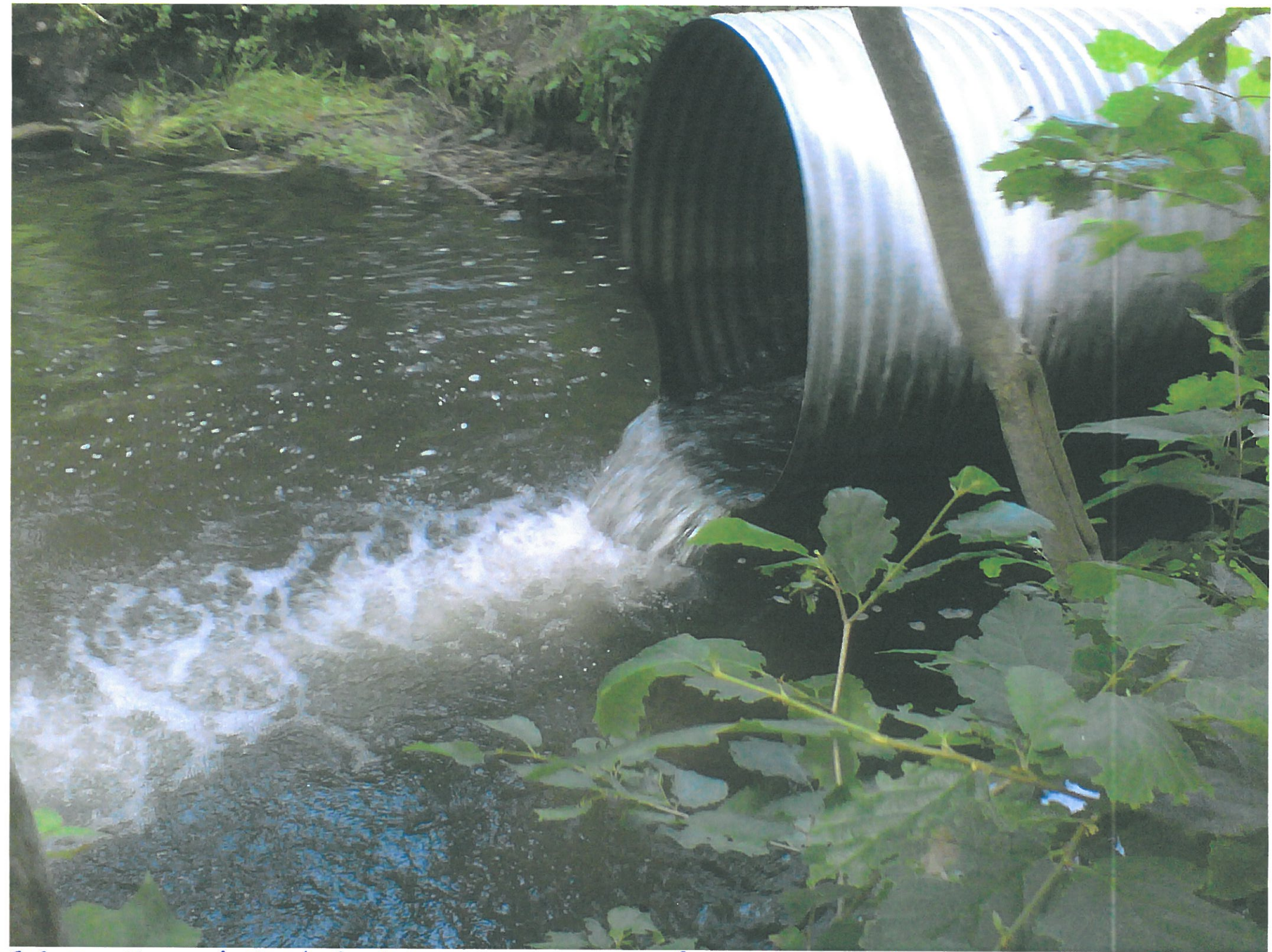
7.3.12 View of Perched Culvert and water fall from S.E. and downstream - Carlton Creek
