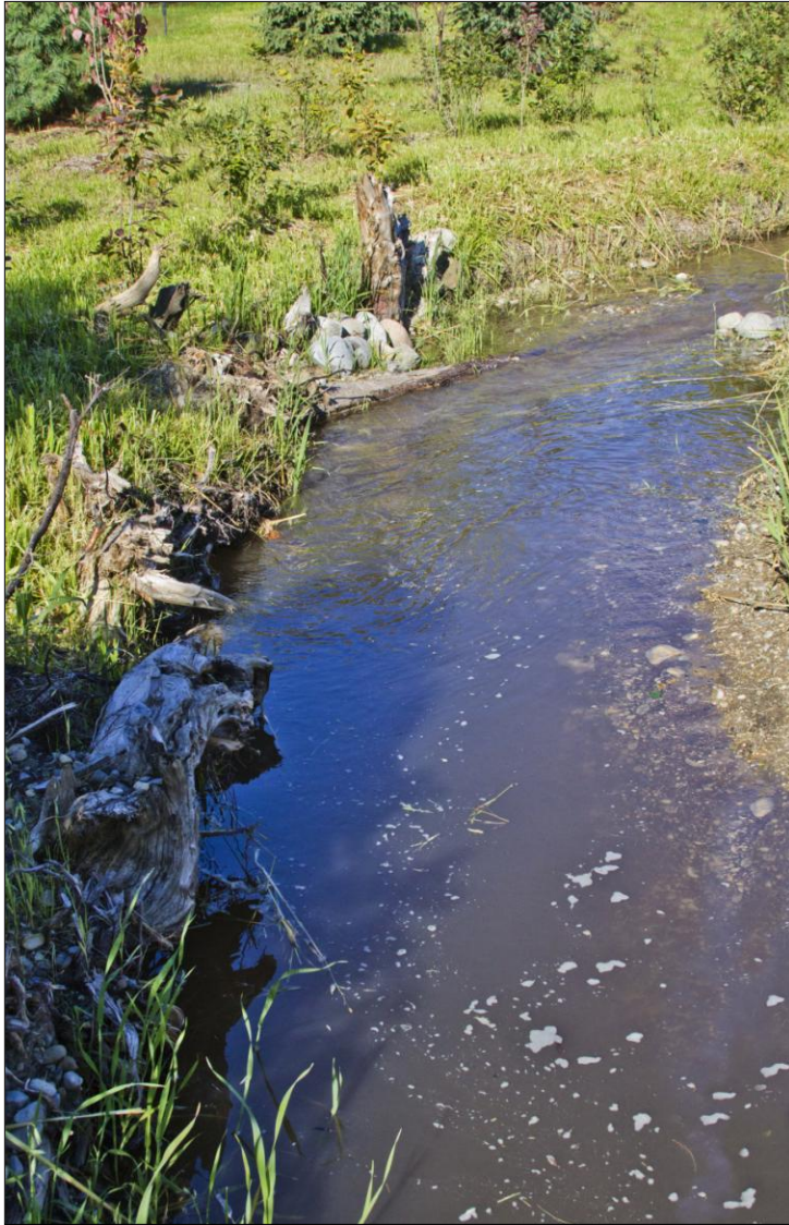
Left: New stream channel just after letting water in (west side of Beaumont Ave crossing)
