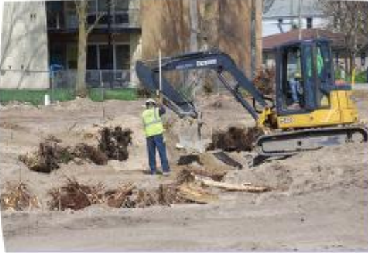
Page 1, clockwise from top left: Kids Creek runs mostly underground near Sixth and Beaumont on the Munson campus. Plans illustrate the stream's new above-ground meandering channel. Logs are put into place to define streambanks. Workers create the new stream bed. This page, clockwise from top left: Workers place root wads to create the new streambank, which prevent erosion and provide fish habitat. Rocks and logs shape the new streambed. Workers install root wads along the sides of the new meandering stream channel. Executive Director Andy Knott and Program Director Sarah U'Ren chat about the project with one of the crews. Photos by Denise Baker.
